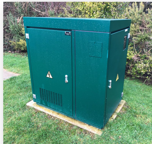
Access (Active) Cabinet
